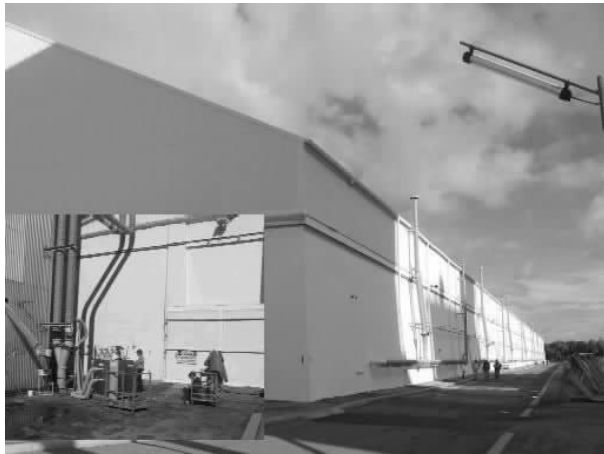
Fig. 2 The 300,000 ton capacity sealed horizontal shed at CBH Kwinana Grain Terminal Western Australia with insert HDS 800/VAPORPH 3 OS fumigation setup.
